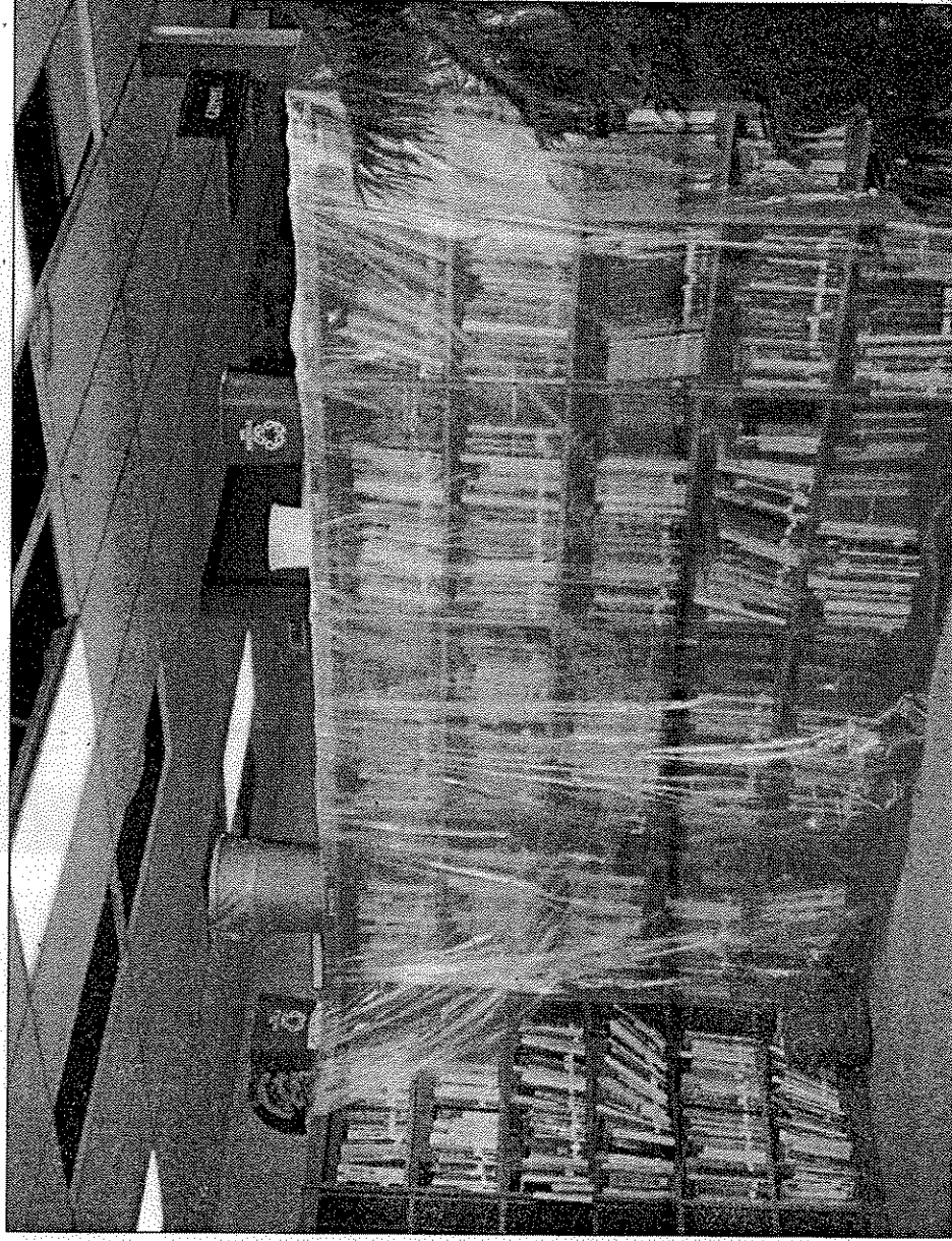
PLASTIC COVERS the books of the Stevens Point Area Senior High School after water leaked from the roof. Buckets have been set up as a temporary remedy to the problem.
