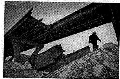
Photo/Gary Porter Judy Grzegorski, safety manager with United Water Services, walks Friday on a pile of gravel that was used to absorb the shock when a 130-foot, 520-ton damaged section of the Hoan Bridge was dropped with the use of explosives Thursday near the Milwaukee Metropolitan Sewerage District plant.
