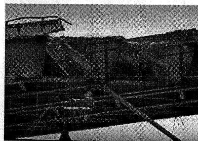
Photo/David Joles Five views of the Hoan Bridge blast and the rubble afterward.
