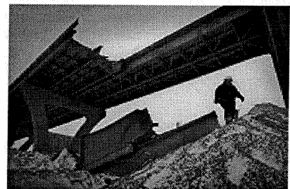
Photo/Gary Porter Judy Grzegorski, safety manager with United Water Services, walks Friday on a pile of gravel that was used to absorb the shock when a 130-foot, 520-ton damaged section of the Hoan Bridge was dropped with the use of explosives Thursday near the Milwaukee Metropolitan Sewerage District plant.
