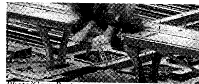
Photo/Gary Porter Aerial view of the damaged section of the northbound span being demolished Dec. 28.
