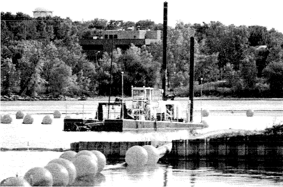
A hydraulic dredge, similar to this one, will be used to remove contaminated sediment in the Little Lake Butte des Morts reach of the Lower Fox River.
