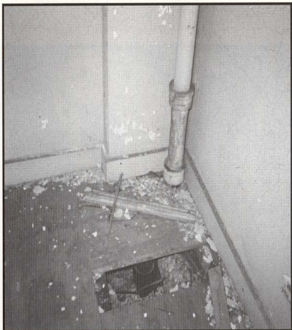
Figure 14.6 Pre-cleaning is needed in areas where contamination and deterioration are high.
