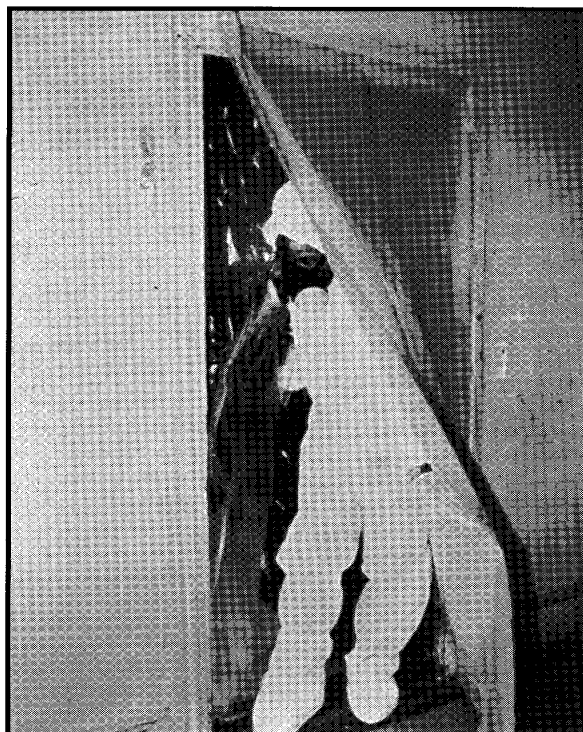
Figure 8.6 Install a Simple Airlock Over a Doorway to Minimize Lead Dust Migration.
