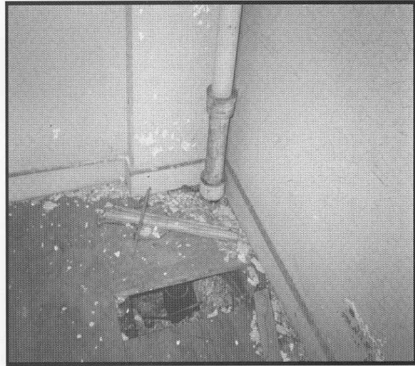
Figure 8.2 Area Should Be Precleaned and Structural Deficiencies in Flooring Repaired Before Lead Hazard Control Begins.
