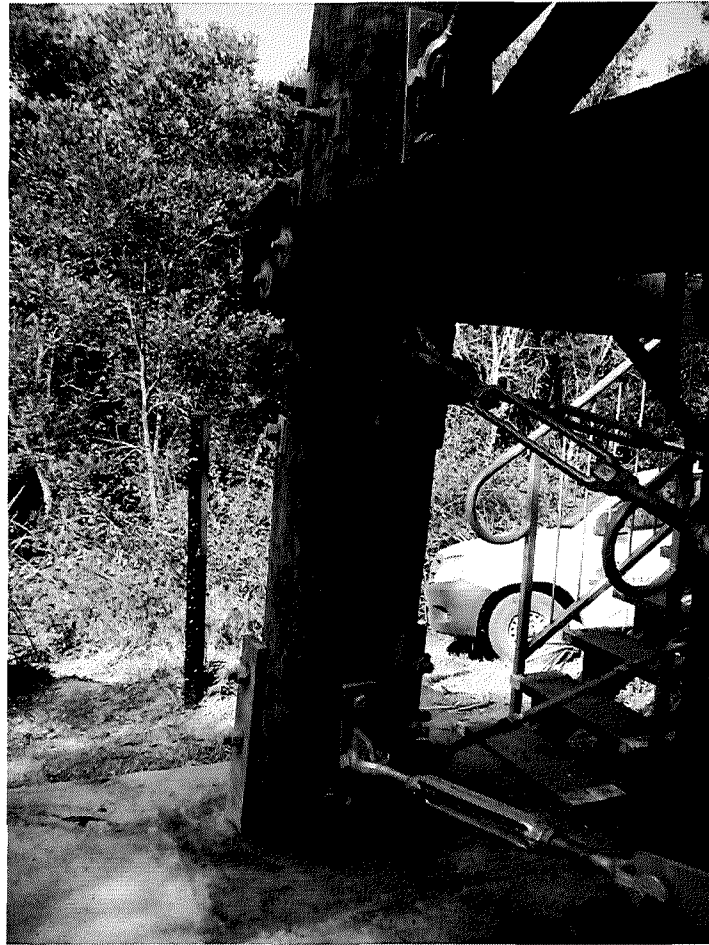
Figure 1-1 Sequence of photos showing segment posting in a column in a timber tower both at the base and mid height. Mt Allen Fire Tower. Decay damage was caused by through brackets and heavy solids painting of the columns as well as embedment in concrete foundations.
