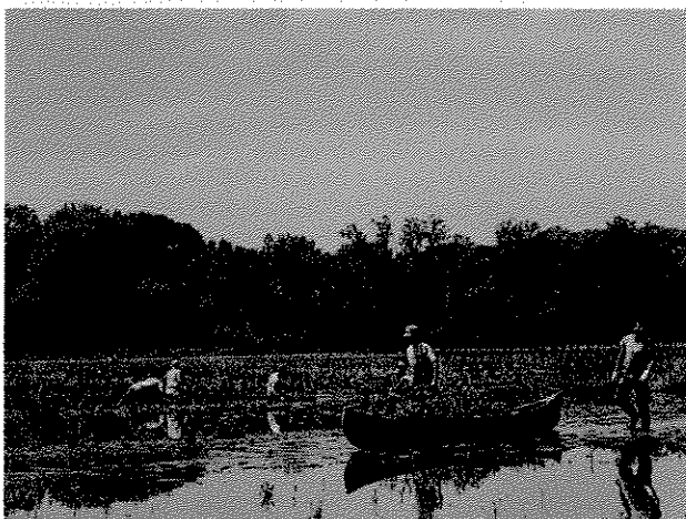
The U.S. Army Corps of Engineers dewatered this freshwater wetland at a restoration site at Kenilworth Marsh in Maryland to facilitate planting. Dewatering was achieved by building temporary dikes made from water-filled tubes designed by the Corps for this purpose. (Photograph courtesy of the U.S. Army Corps of Engineers.)
