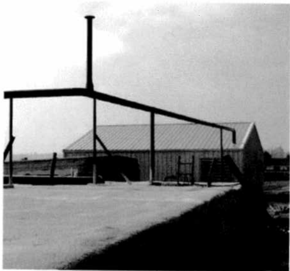
The new digester at Vander Haak Dairy in Lynden, Washington will process manure and wastewater — facilitating growth of acid forming bacteria in the first stage and converting volatile fatty acids into biogas during the second stage for use as heat and power.
