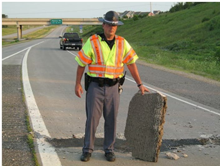
Wisconsin State Patrol NW Region Trooper Robert Unruh handles a chunk of concrete displaced by road buckling.
