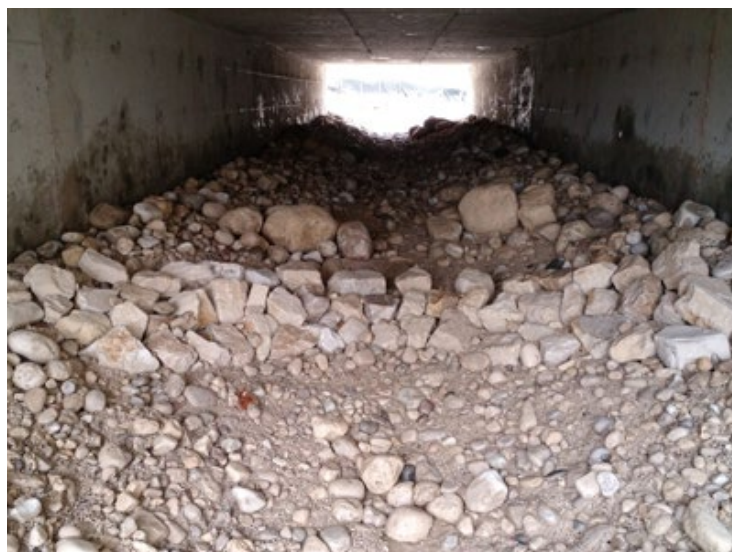
The "riffle, run, pool" zone layout started upstream and continued through the culvert, creating a more natural flow.
