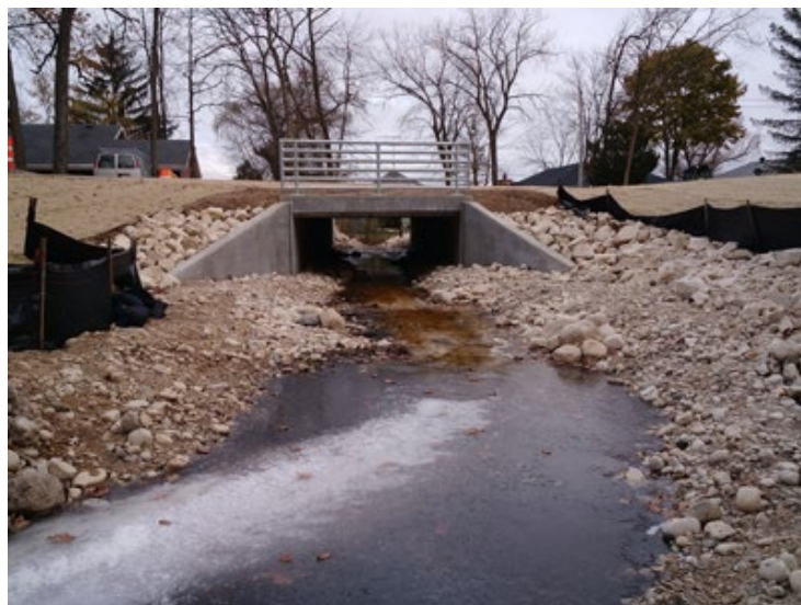
Since the project's completion in mid-November, fish have been spotted upstream of WIS 67. The box culvert opened the stream to a more natural flow, allowing fish to reach traditional spawning grounds.
