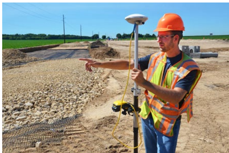
Southwest Region Project Development Section Engineer Greg Payne uses a mobile GPS to verify design information on a recent project.
