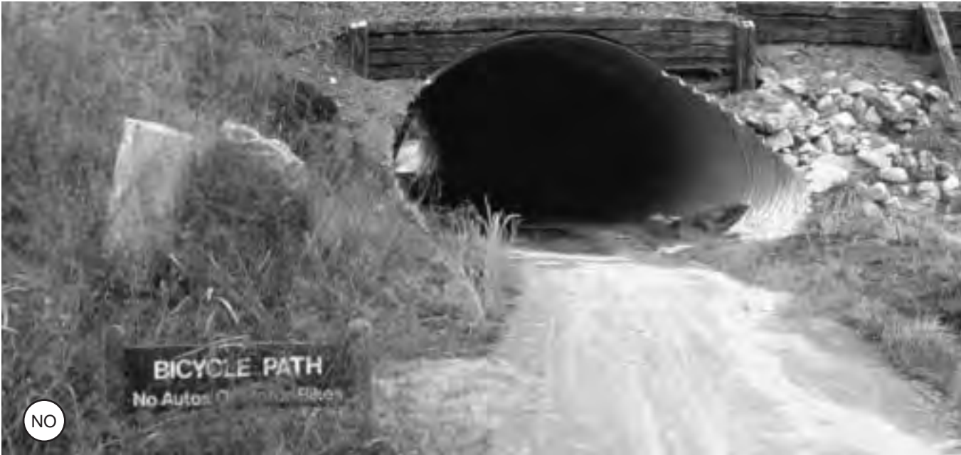
Figure 4-50: Path lighting is particularly important where ambient light levels change dramatically, as in an underpass.
