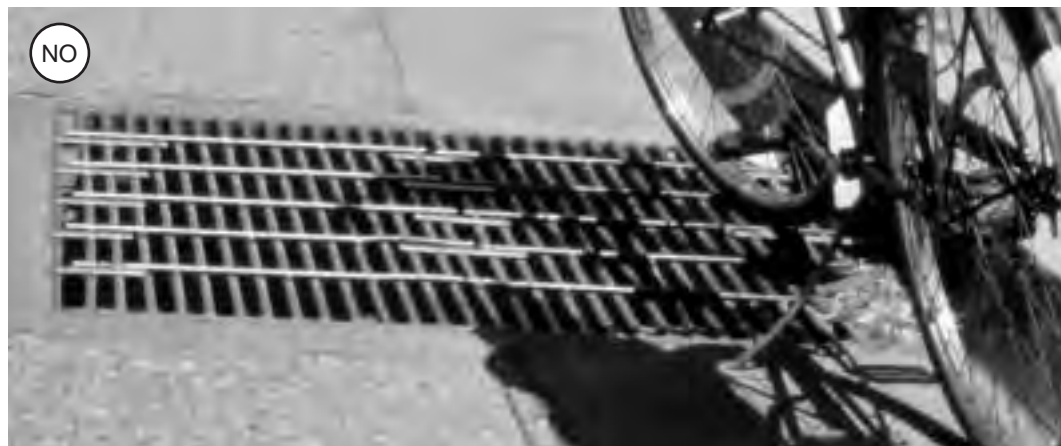
Figure 2-21: Temporary measures, like welded straps, may be more costly in the long run.
