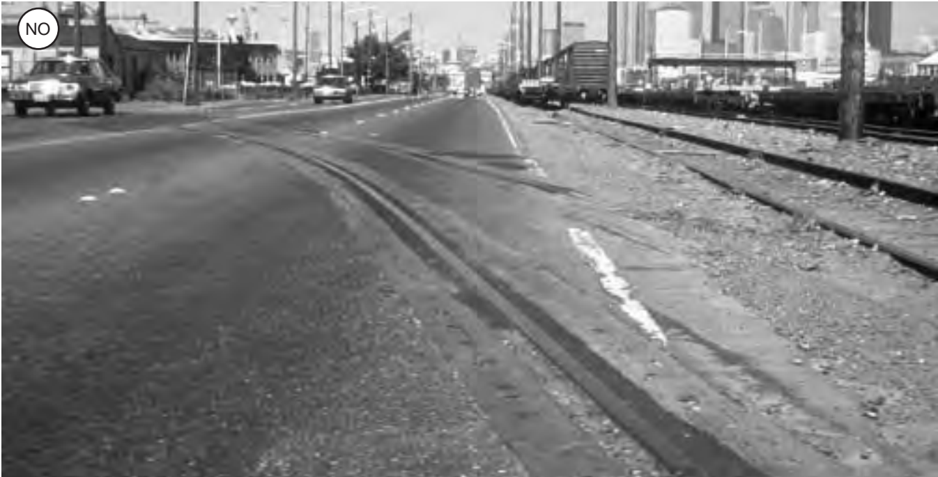
Fig. 2-38: An old unused diagonal railroad crossing. The flangeway can catch and turn a bicyclist's front wheel, especially when wet, and the roughness can also cause a tumble.
