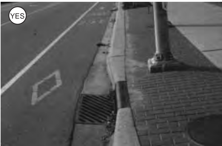
Figure 3-13: A drain inset into a 1ft. curb head provides extra space in tight places.
