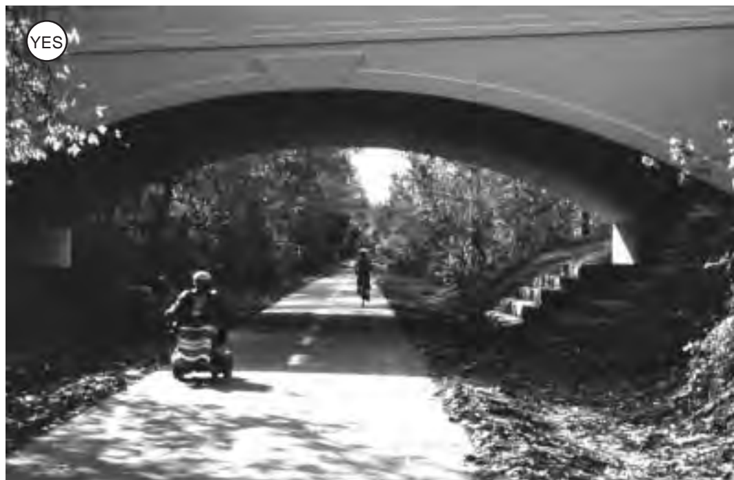
Figure 4-117: An open and airy underpass. Note the generous clearances on either side.
