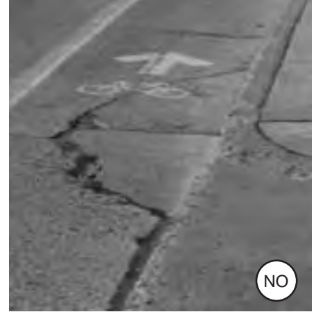
Fig. 3-11: Serious pavement cracks in a bicycle lane can cause a bicyclist's front wheel to turn, resulting in a crash.
