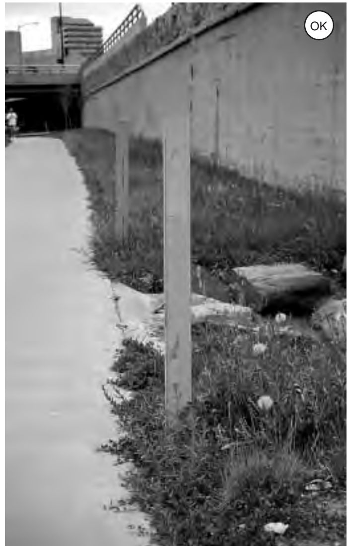
Figure 4-49: Hazard markers identify drainage structure adjacent to the path edge. If possible, such structures should be offset at least 3 feet from the edge of the path and covered with a bicycle-safe grate.
