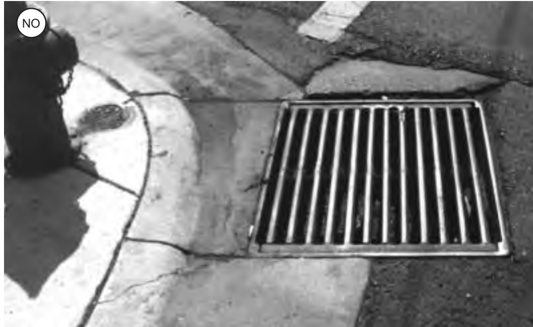
Figure 2-14: This drainage grate has two main problems. First, its parallel bars and slots can trap a bike wheel. Second, it's located in a likely path of a turning bicyclist.
