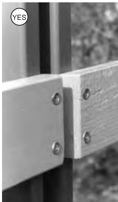
Figure 4-121: A simple rub rail mounted at handlebar height can divert out-of-control bicyclists back onto the pathway.
