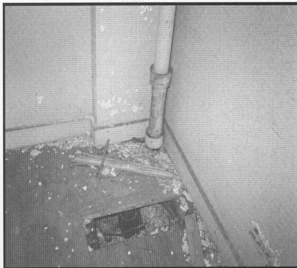
Figure 8.2 Area Should Be Precleaned and Structural Deficiencies in Flooring Repaired Before Lead Hazard Control Begins.
