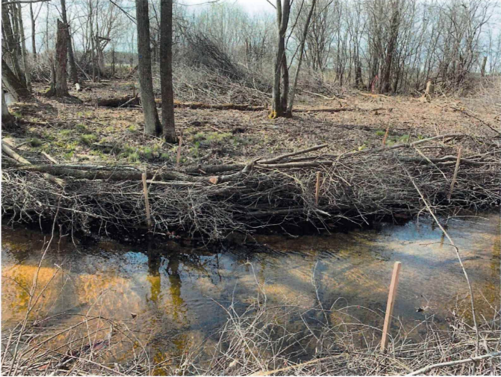
Figure 5. Brush bundles are placed along banks of the river to promote natural narrowing and deepening of the channel. A narrower and deeper channel helps improve floodplain connectivity, wetland conditions, and native brook trout habitat.
