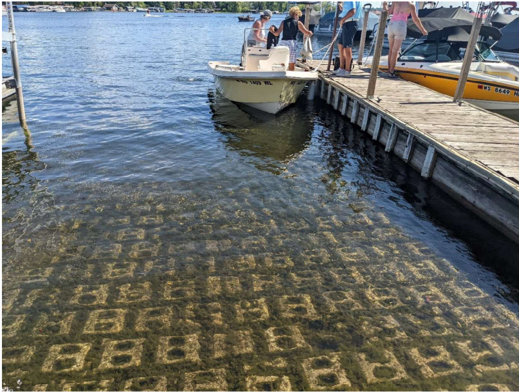
Existing conditions – eroding cinderblock launch.
