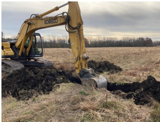
An excavator disabling drainage tile at the Meachem Road ILF site in Racine County.
