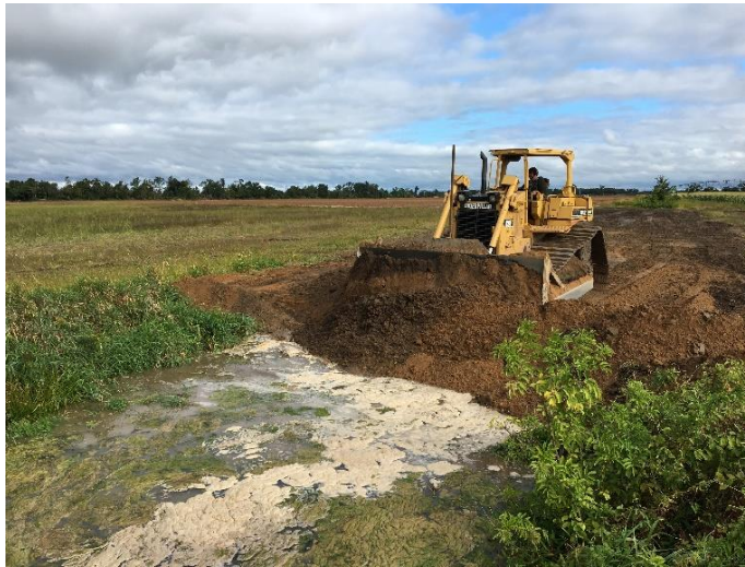
The filling of drainage ditches to restore wetland hydrology at the Plover Soik ILF project.
