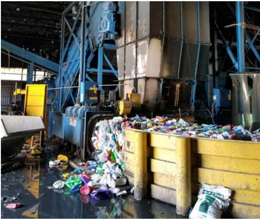
The aftermath of a major fire in May 2023 at the Milwaukee materials recovery facility. While the exact cause of this fire is unknown, a lithium-ion battery is suspected. Photo courtesy city of Milwaukee.
