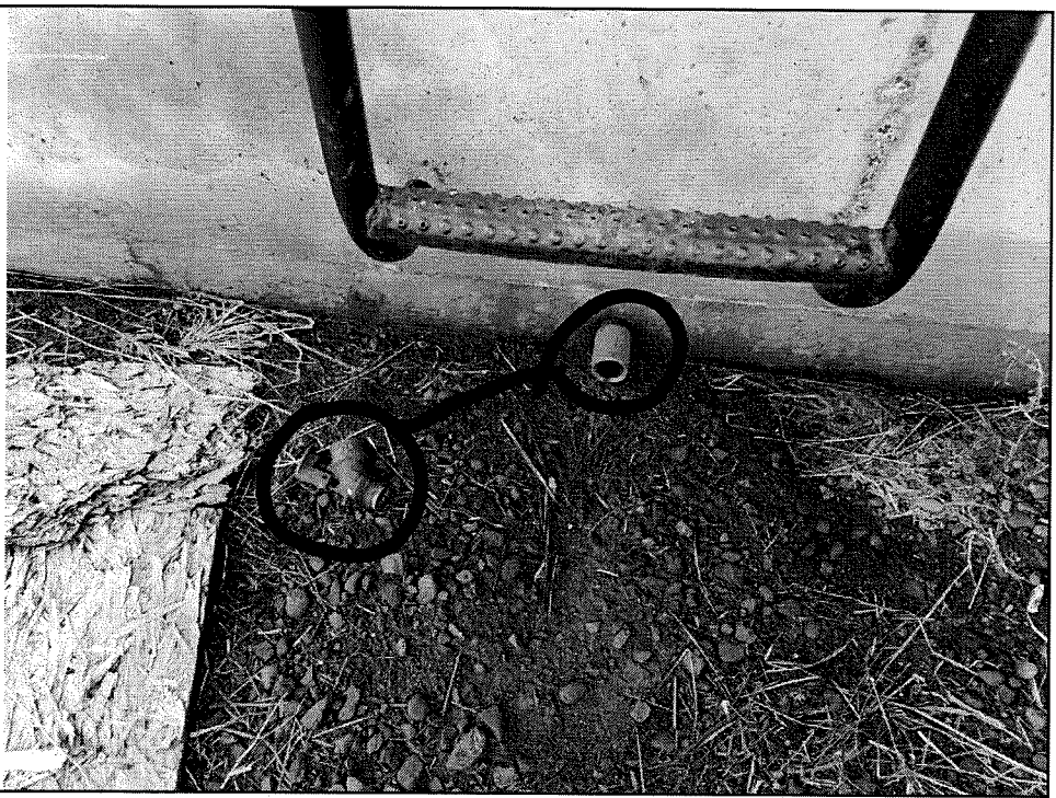
Containment not plugged allowing for contamination to seep into earth
